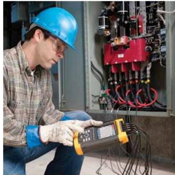
Measure all power parameters, find events and anomalies in seconds
